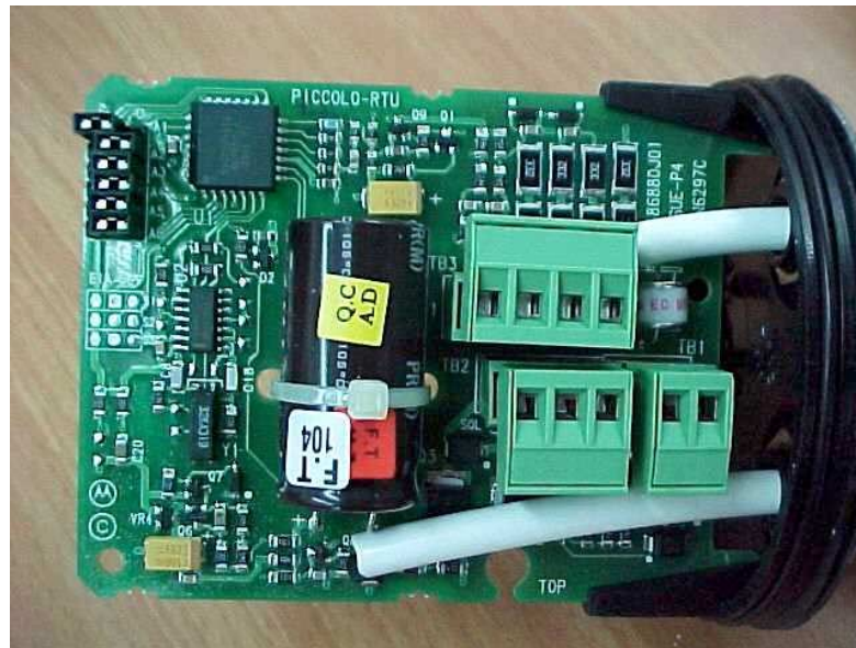
Fig. 5 Internal view of Sample 1 after water test (no traces of water observed)
