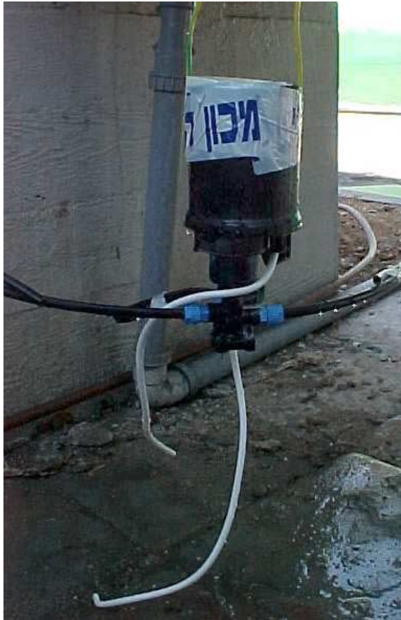
Fig. 4 Water test set-up
